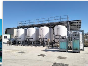
Siciliacque: Trapani desalination plant
